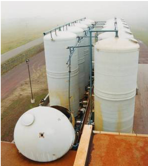
Fig. 9. Collapsed tank in tank farm.
