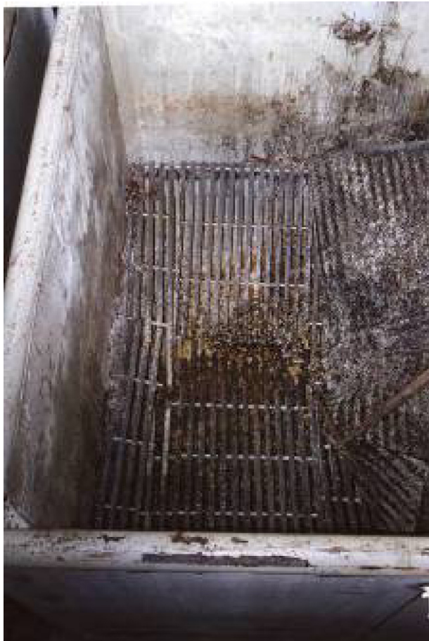
Fig. 4. Grating beams fractured at mid-span in biological media chambers.
